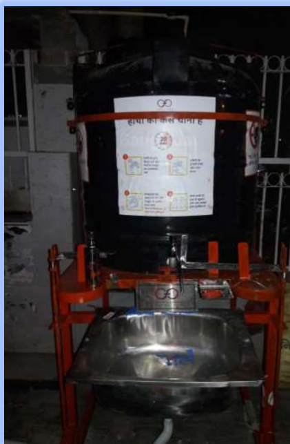
Handwashing station installed at Laxmi Narayan Mandir, Sarita Vihar in south-east Delhi
