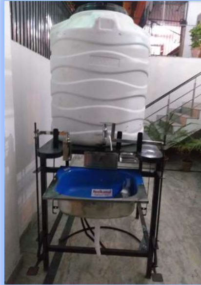
Handwashing station installed at the MP office in Jagriti Enclave, Vikas Marg, in east Delhi
